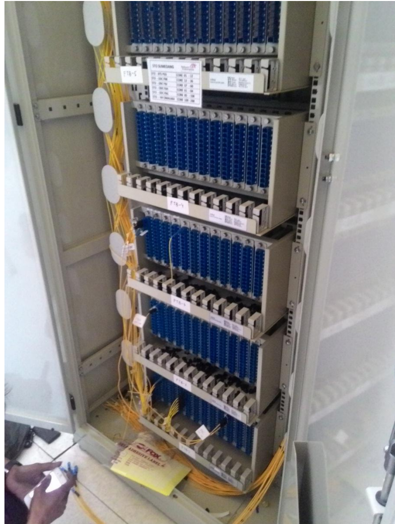
Gambar 8 Fiber Termination Management (FTM)
